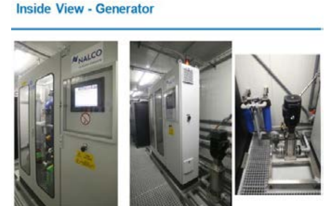
Figure 36: Inside view of the system
