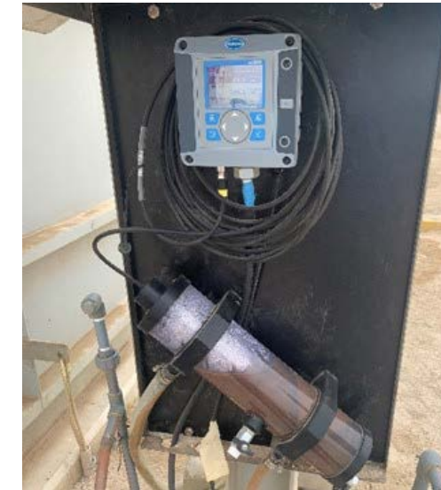
Figure 40: Ammonium and nitrate probe analyzer, By: Abdulaziz Ghowainem, onsite photo at Seawater water injection plant
