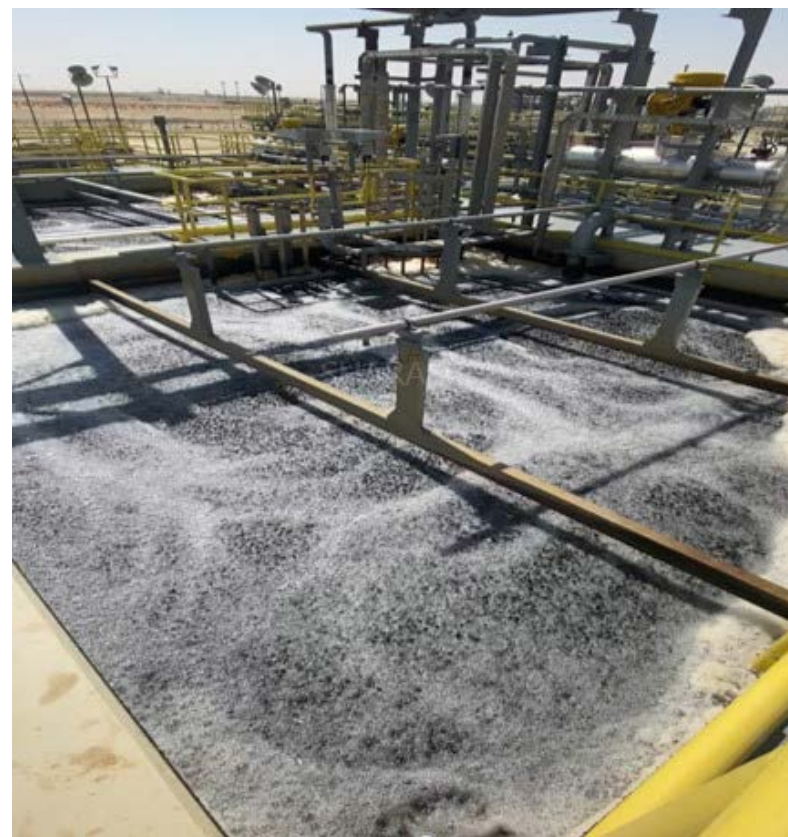
Figure 8: FGP Moving Bed Biofilm Reactor
